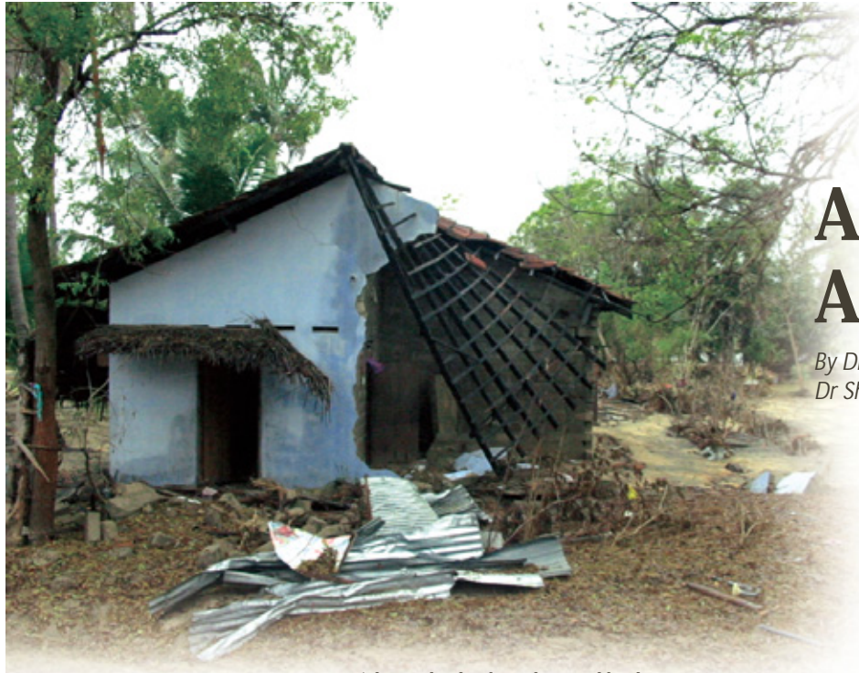
A house that has been destroyed by the tsunami.
